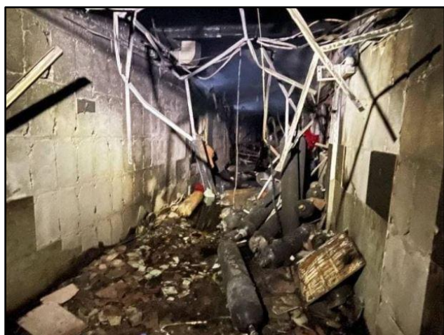
Figure 13. Comprehensive destruction of oxygen systems.
