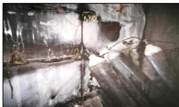
Figure 6. Fire and explosion in oxygen cylinder filling unit.
